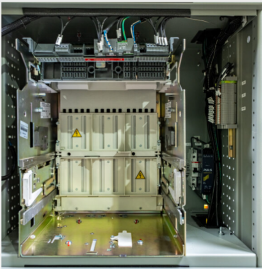
Breaker Compartment with Vertical Wireway
