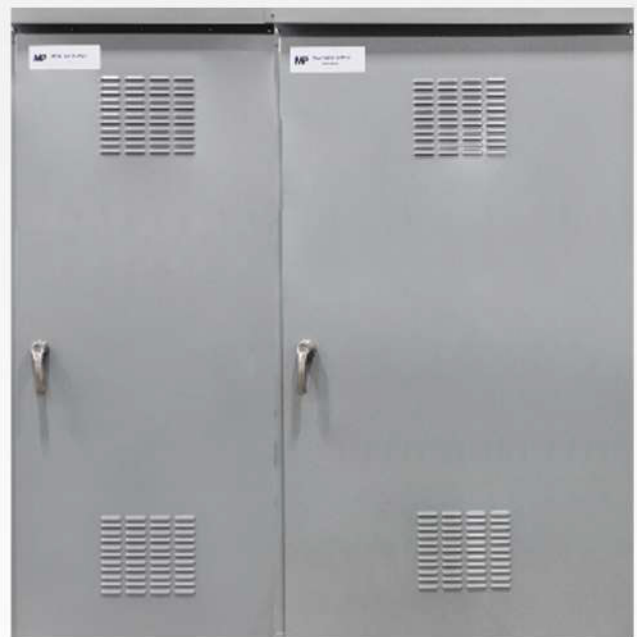
NEMA 3R Switchboard
