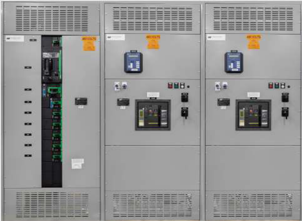
Main-Gen Switchboard with ATS Controller
